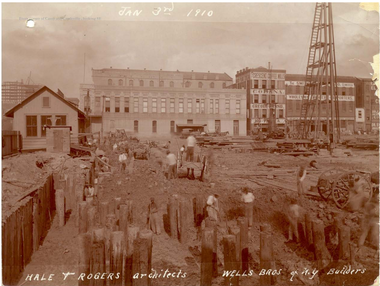
1910 excavation of basement and driving of pilings at 600 Camp; photo courtesy Court of Appeals.
