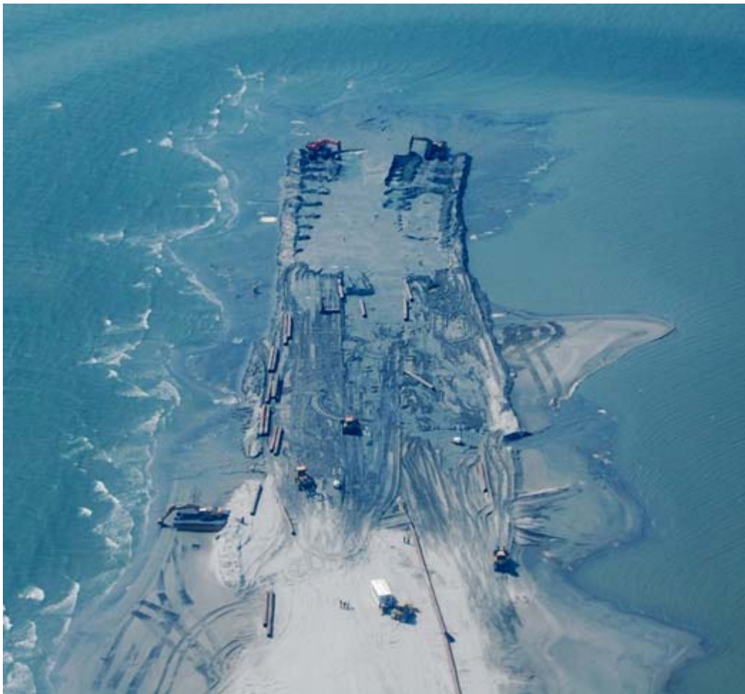
Sand berms under construction by the State of Louisiana, summer 2010. [Photograph: Josh Lewis, special thanks to Tor Tornqvist]
