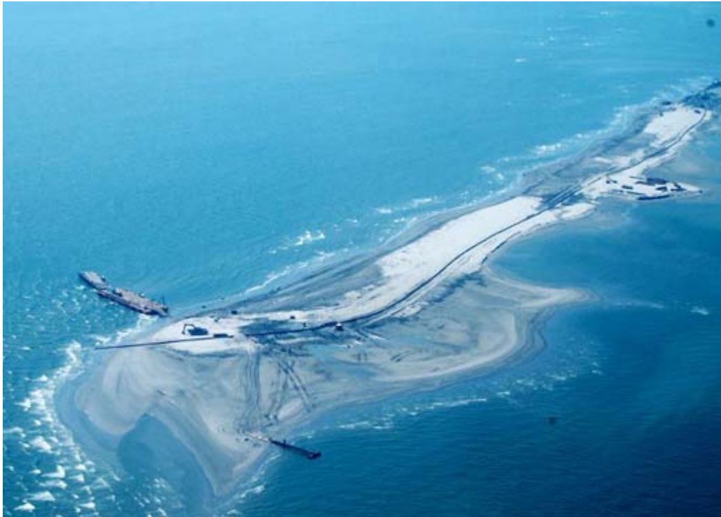
Sand berms under construction by the State of Louisiana, summer 2010, in a desperate but dubious attempt to prevent BP's oil from reaching shore. [Photograph: Josh Lewis, special thanks to Tor Tornqvist]
