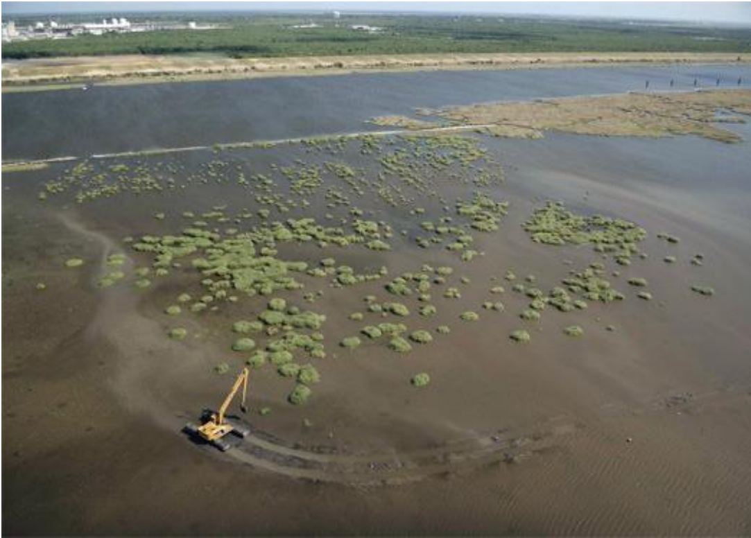
Beneficial use of dredged sediment east of the Inner Harbor Navigation Canal Lake Borgne Surge Barrier, New Orleans. [Photo by USACE]
